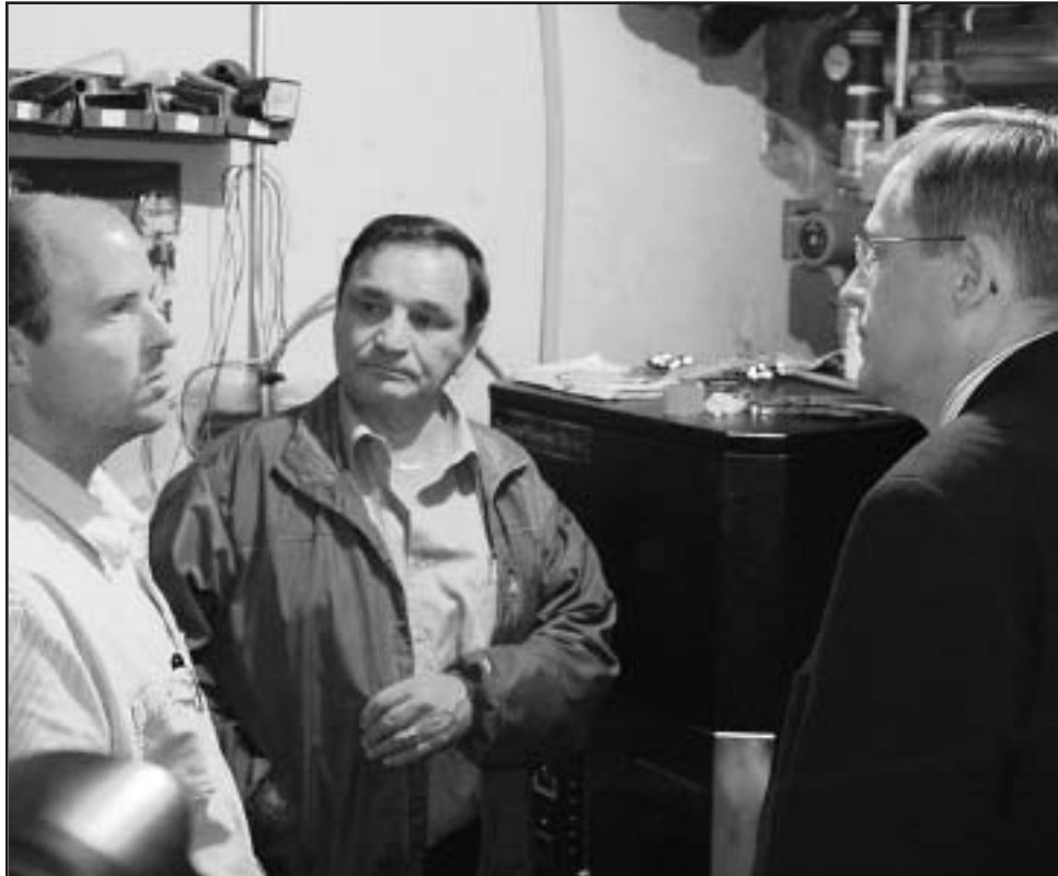
Jim Durocher, President of SaskNative Rentals and Justice Minister Frank Quennell get a lesson in operations from Brent Bedrock of Gibson Heating of a newly installed boiler in an affordable housing apartment on Idylwyld in Saskatoon.
